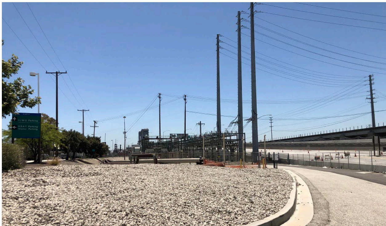
Distribution Station No. 119 from north (May 13, 2022 photo)
