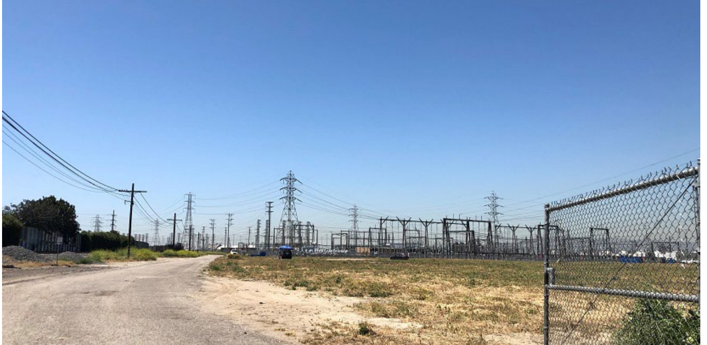
SCE Hinson substation from north (May 13, 2022 photo)
