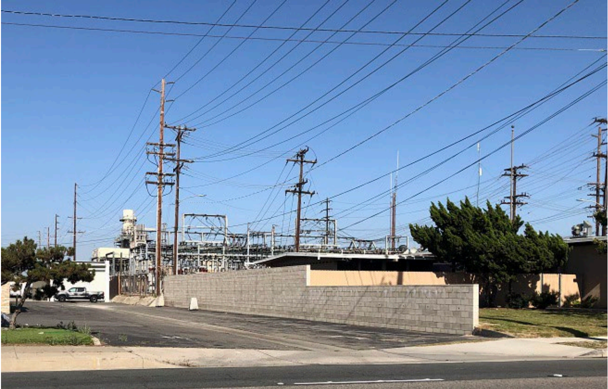
APU Dowling Sub (May 4, 2022 photo)
