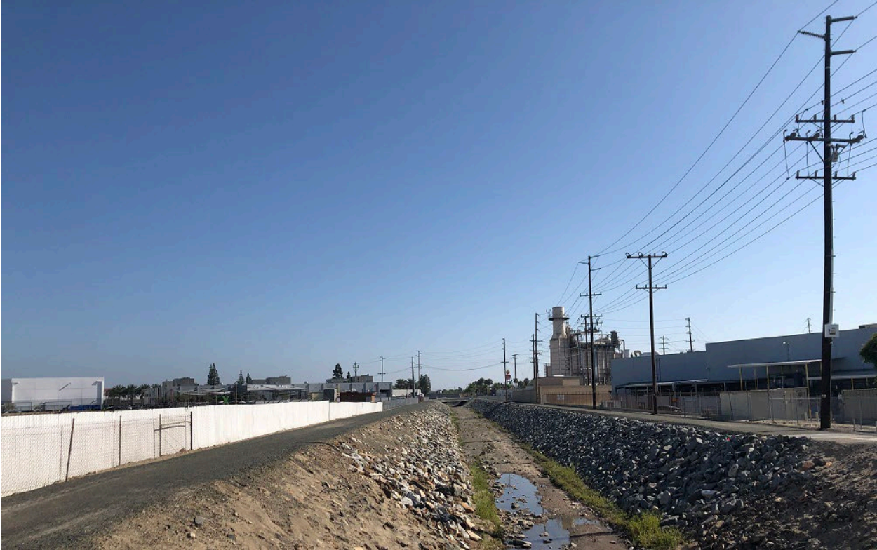
Looking south along Carbon Canyon Diversion Channel and 69 kV APU overhead line towards APU Dowling Sub (May 4, 2022 photo)
