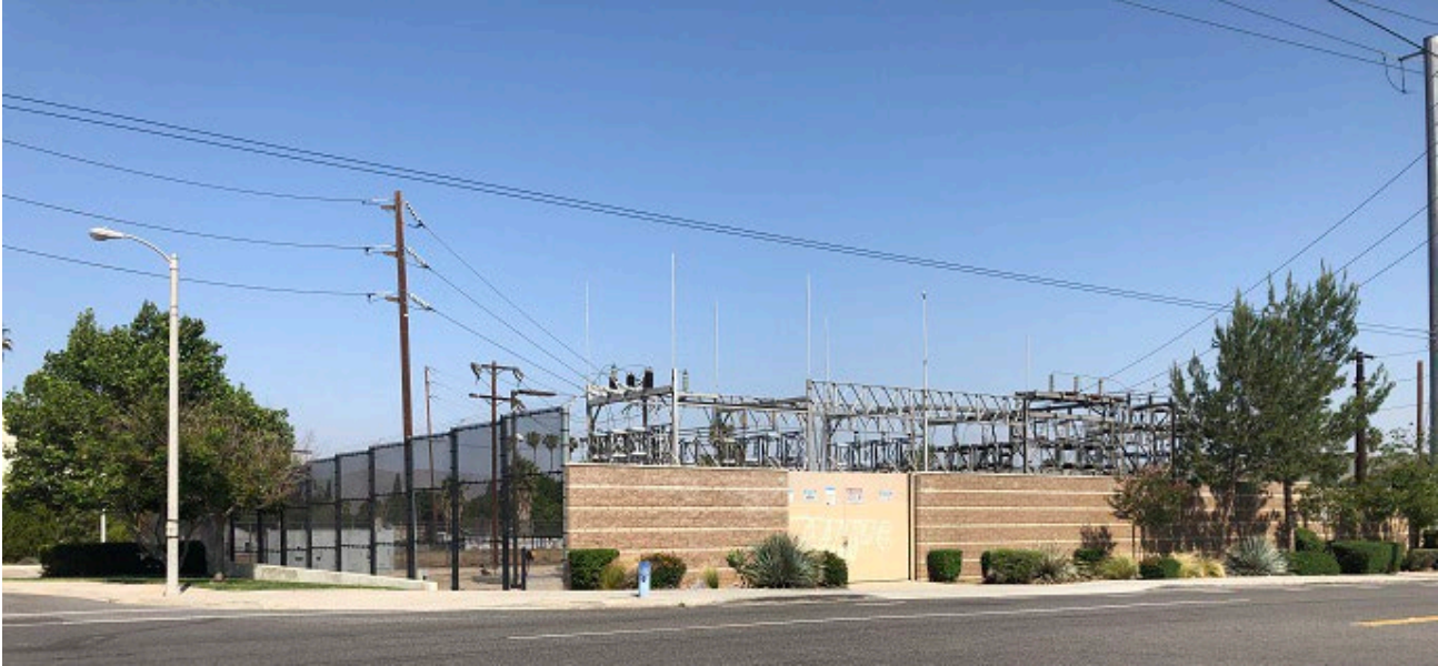
RPU Hunter Substation (May 1, 2022 photo)
